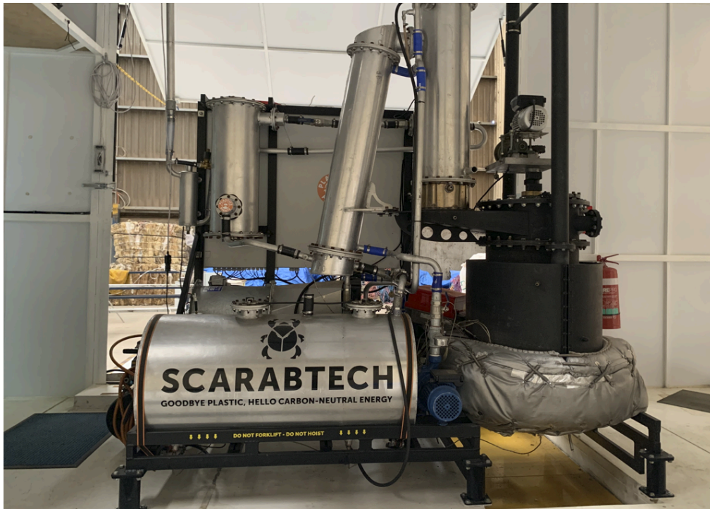
Pyrolysis unit inside purpose-built trailer for easy transport.
